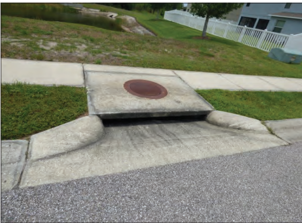
Stormwater Drainage Curb Inlet
