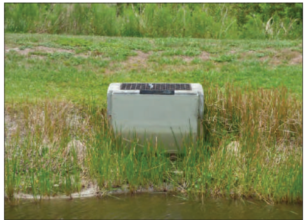
Stormwater Drainage Control Structure
