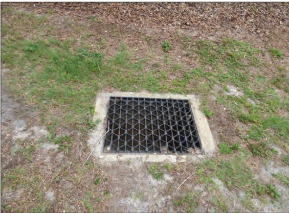
Stormwater Drainage Grate Inlet
